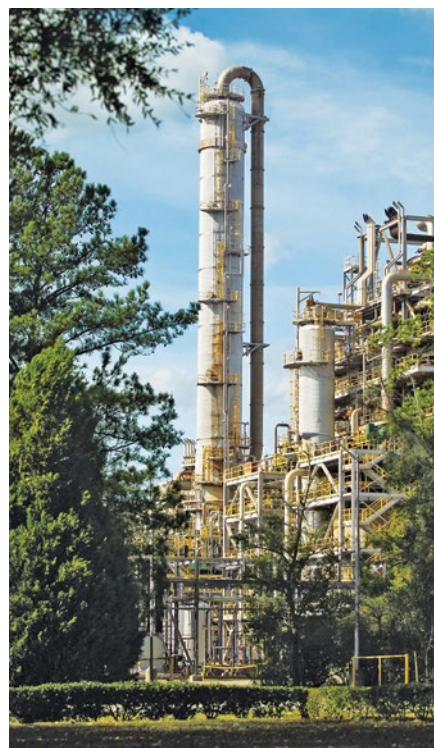
The dehydration tower at BP's South Carolina purified terephthalic acid plant
